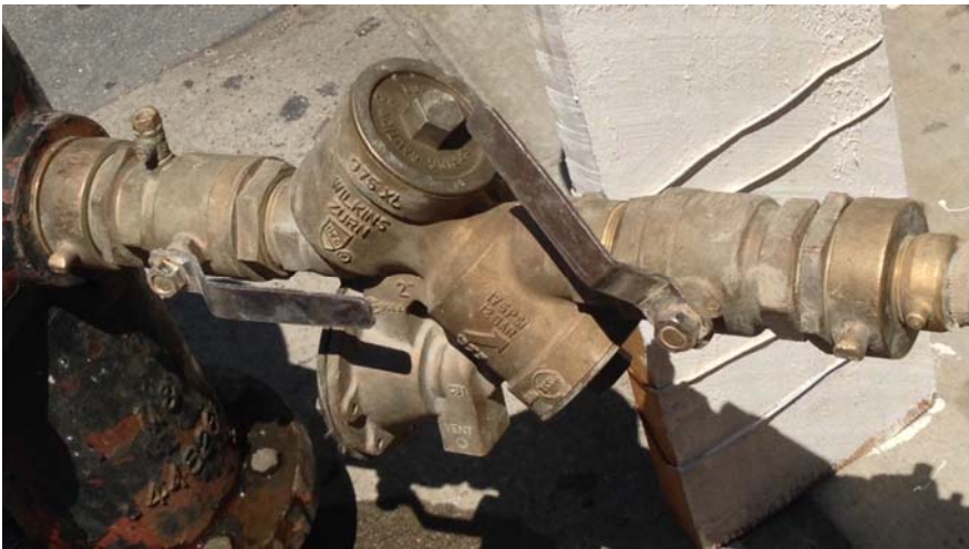
Backflow Prevention Device
